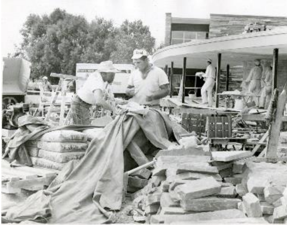
Construction workers busy at the Harvest House in July of 1958. Piles of local sandstone are pictured in the foreground. Carnegie Library for Local History/Boulder Daily Camera Collection.
