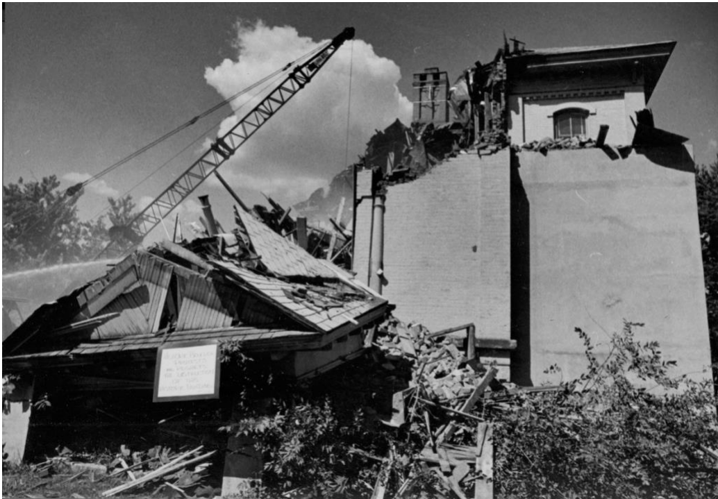
Demolition of Central School. On a portion of the roof which fell to the ground was the sign, "Historic Boulder Protests and Regrets the Destruction of this Historic Building." Carnegie Library for Local History/ Town & Country Review Collection.
