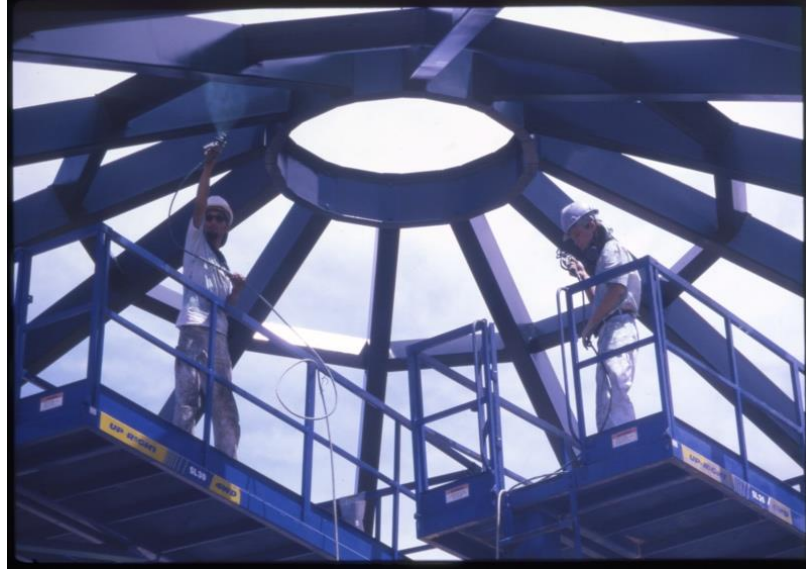
Construction on the pavilion at the Regal Harvest House Hotel in 1997. Carnegie Library for Local History/Boulder Daily Camera Collection.
